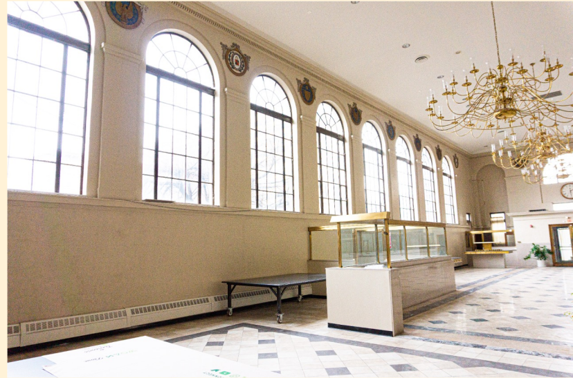
Replace Cracked & Missing Windows
